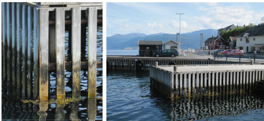
Fig. 5.9 Wooden pier exposed to fluctuations of the water level. Image courtesy of Lone Ross Gobakken, NIBIO
