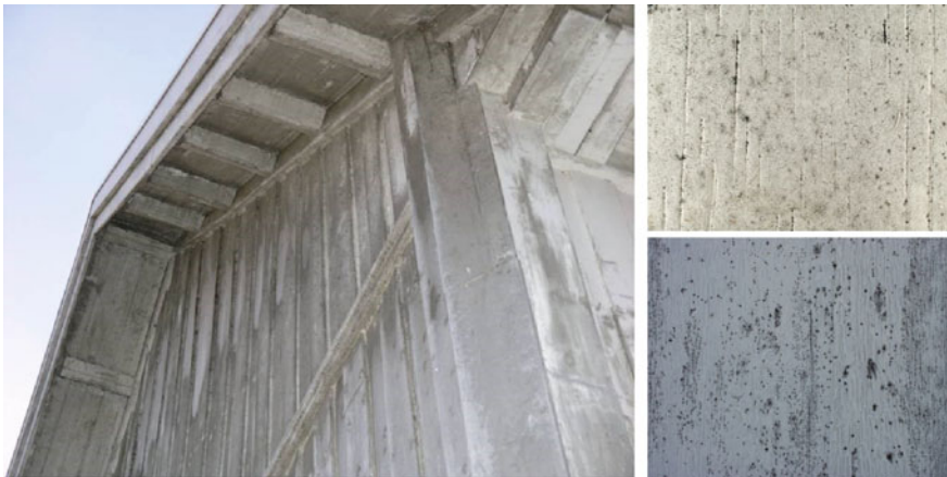
Fig. 5.5 Wooden façade with the signs of moulds growth. Images courtesy of Lone Ross Gobakken, NIBIO
