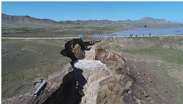
Figure 3. Final breach of Zenglongchang dam.
