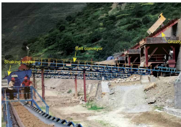
Figure 14. Screening system for the PBG dam (at the courtesy of Yao FH).
