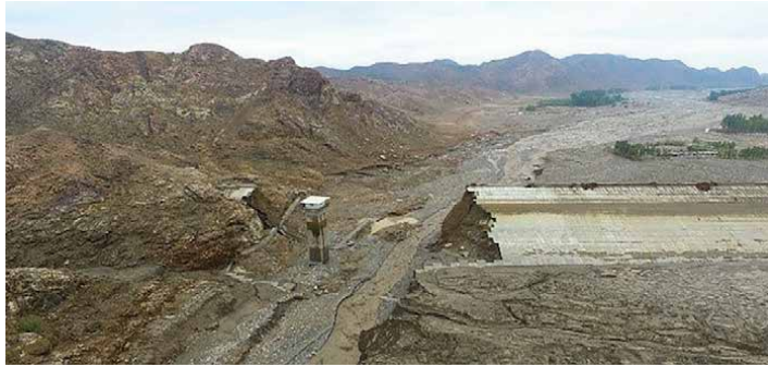
Figure 4. Final breach of Sheyuegou dam.
