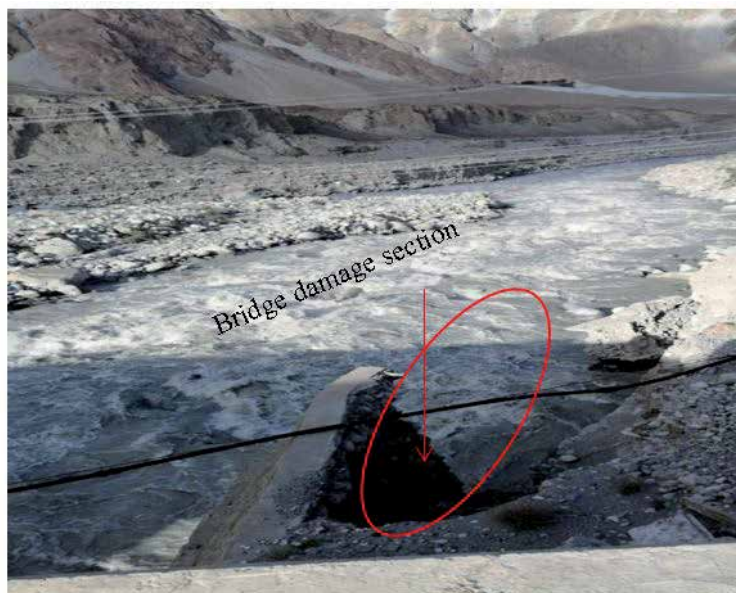
Figure 9. Impact of high flow of Batura glacier on CPEC bridge.
