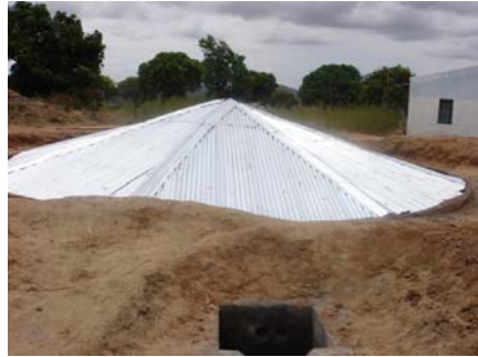
Figure 11.7 Underground tank (150,000 liters). (Source: Author's own).
