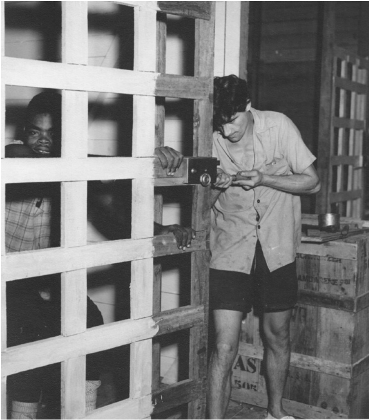
ILLUSTRATION 44 The carpenter Erwin Mathis renovating what might be a psychiatric cell, early 1950s
