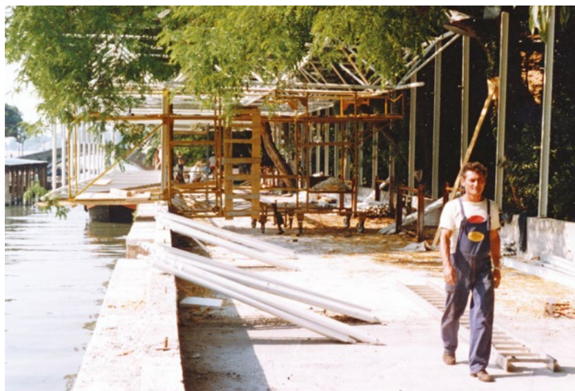
Venice Biennale: The Australian pavilion under construction shortly before the vernissage. Even though the pavilion was still not weatherproof the show was installed anyway for the duration of the vernissage before being dismantled until the building was completed Image from author’s archive
