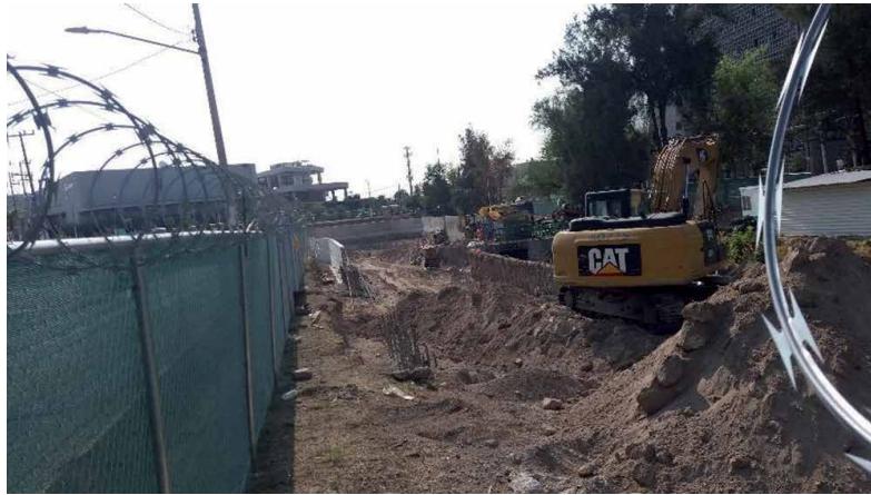
Figure 18. Construction of a dam clothes to Plaza Patria mall, this for contain the rains in the high side of the basin. Source: Jorge Navarro personal files.
