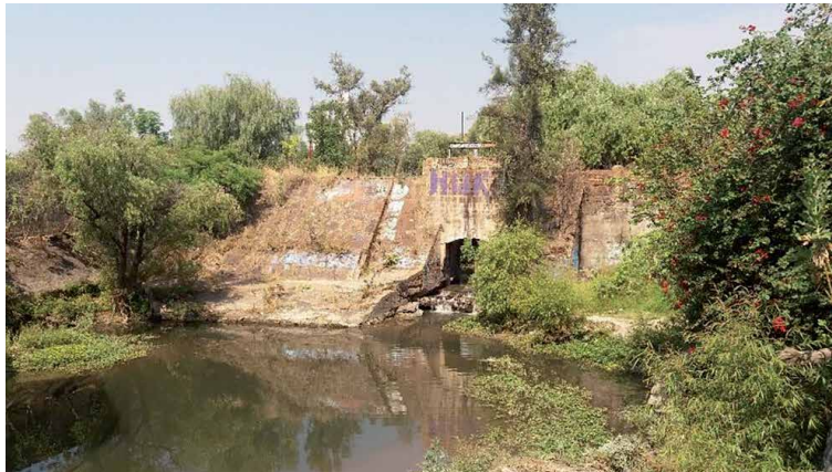
Figure 19. Zoquipan dam, in the past, the water conserved make the energy in Atemajac Factory, today is abandoned. Source: Jorge Navarro personal files.
