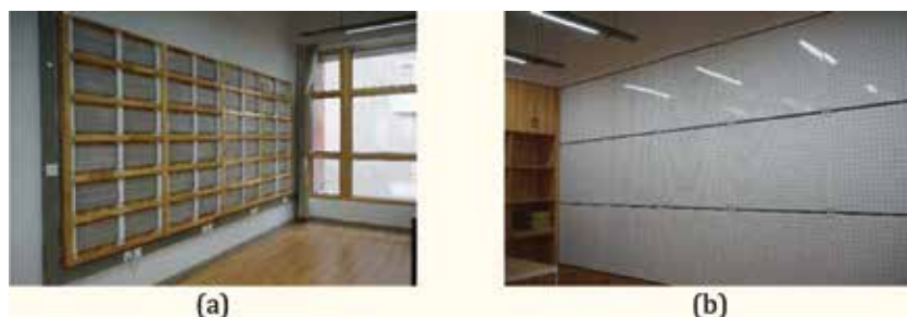
Figure 17. Actual installation effect of the PCM panel: (a) exposed to indoor air and (b) decorated with perforated aluminum plate.
