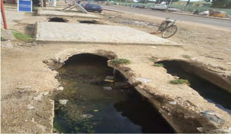
Fig. 7 Poor drainage filled up with silt, obstructing the free flow of storm water along Dala Orthopaedics Gwammaja. (Source: Field Survey 2019)
