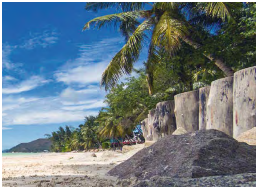
Fig. 5 Timber piling for coastal protection on Praslin Island (World Bank and MEECC 2019)
