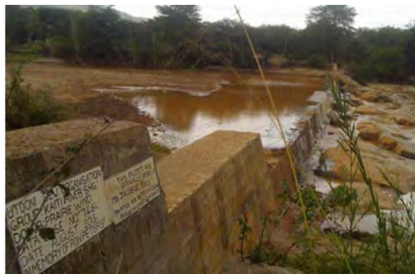
Fig. 13 A sand storage dam construction in Makueni County during the dry season (Photo taken by Mary)
