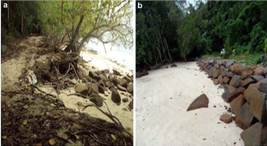
Fig. 4 Severe erosion at Anse Marie-Louise on Praslin Island highlighting coastal erosion (a) and the construction of rock armoring (b) to mitigate the impacts of coastal erosion (MEECC 2019)
