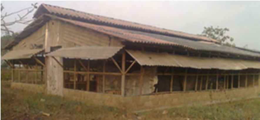
Fig. 3 Low-walled broiler housing units
