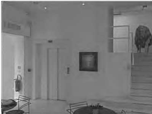
Figure 8: An inaccessible lift
