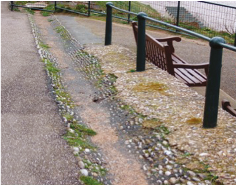
Figure 13.3a Budleigh Salterton seafront: drainage guttering (Source: author)
