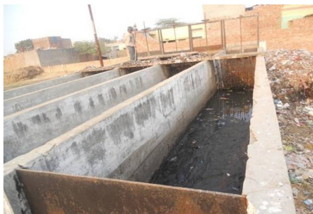
Figure 8.12 Poor maintenance of the primary treatment unit prior to WSP in the Municipal WWTP in City of Agra.
