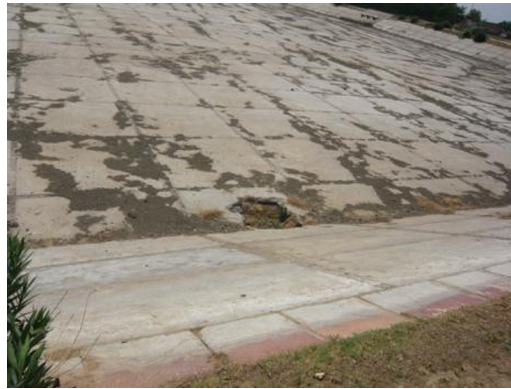
Figure 17.4 Hole in lining of facultative anearobic pond.
