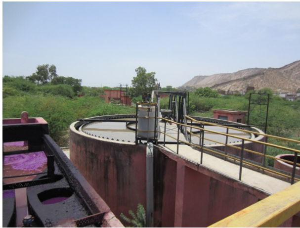
Figure 10.3 Removal of phosphorus using lime precipitation technology (first step in tertiary treatment).
