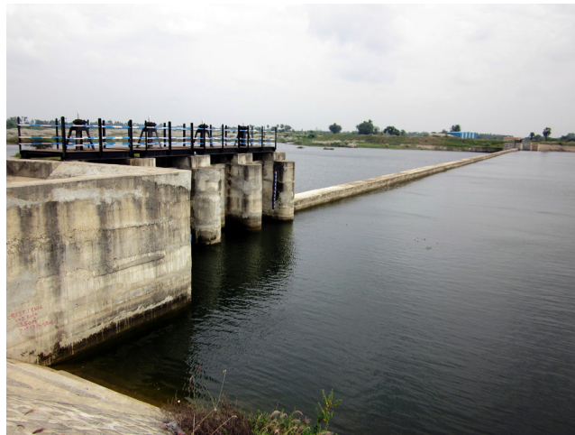
Figure 16.5 Paleshwaram check dam across Arani River, north of Chennai, Tamil Nadu, India (Photo: S. Parimala Renganayaki, Anna University, Chennai).
