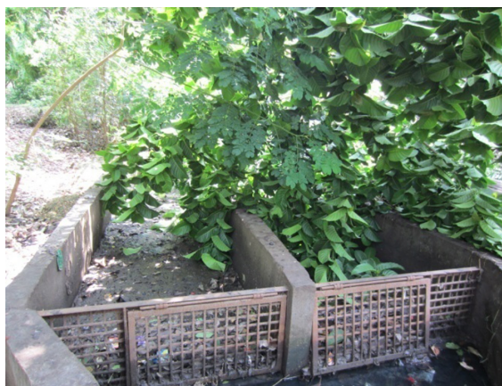
Figure 8.6 Poor maintenance of the primary treatment unit prior to HSSF-CW in Ekant Park, City of Bhopal, central India.
