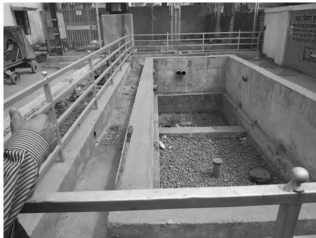
Figure 5.4 Recharge pit at Raipur Municipal Corporation headquarters (Source: Raipur Municipal Corporation).
