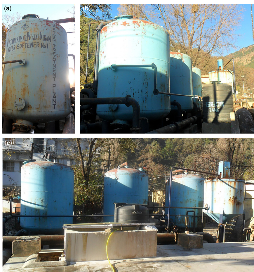
Figure 12.2 Ion-exchange water softening system treating bank filtrate at Nainital.
