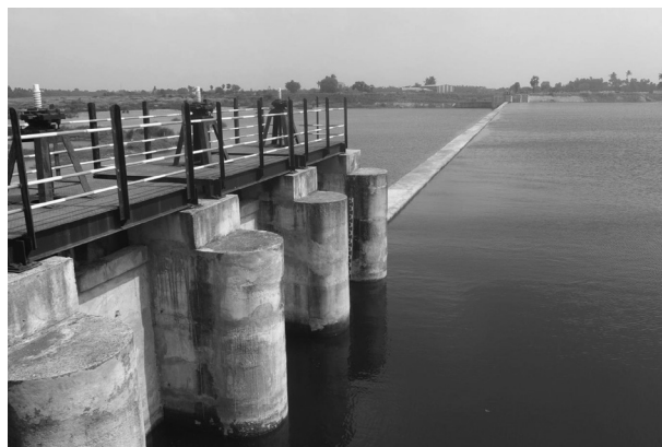
Figure 5.2 Check dam in Araniyar River in Tamil Nadu (Source: Christoph Sprenger).
