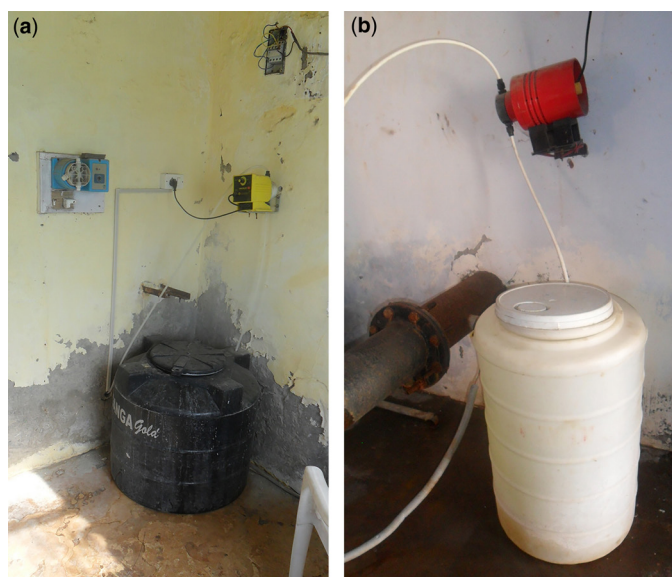
Figure 12.1 Typical sodium hypochlorite dosing system for RBF wells in Haridwar.
