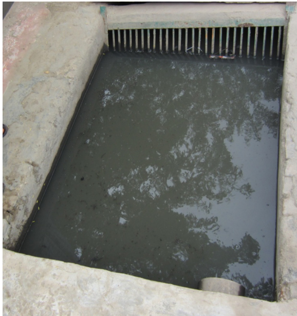
Figure 10.7 Pre-treatment unit comprising of bar-screen and grit removal.
