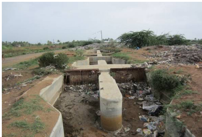
Figure 8.13 Poor maintenance of the primary treatment unit prior to WSP in the Municipal WWTP in City of Miraj, western India.
