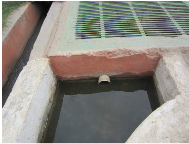
Figure 10.10 Tank for collection of treated wastewater to be sent for gardening and irrigation.
