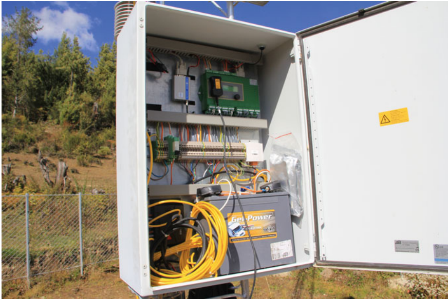
Fig. 2.3 Rara Nepal. OTT data logger and data transmission modem in IP65 enclosure
