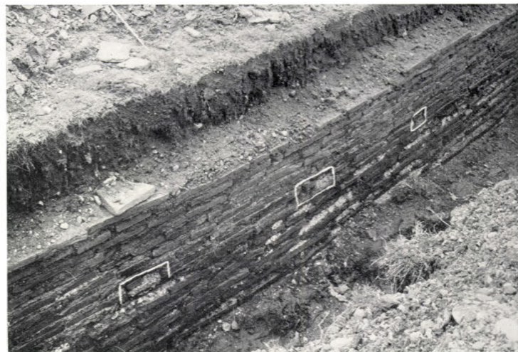
B. Drain, showing difference between upper and lower parts, and line of holes filled with mortar. [39], p. 88.
