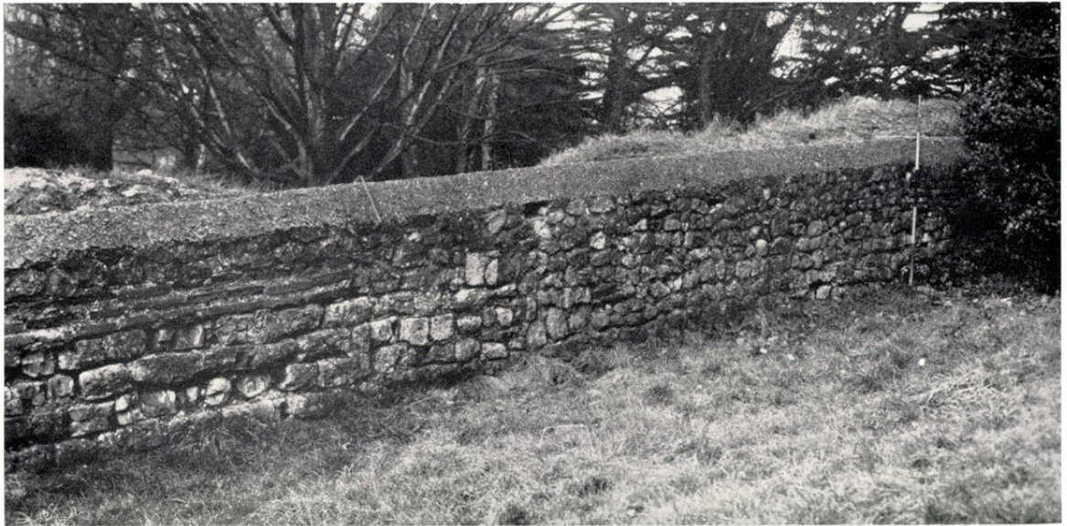
A. Inner face of town wall in Castle Park, showing face repaired where tower was removed. p. 35.
