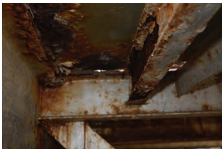
Figure 8. Significant deterioration of bridge structural members.
