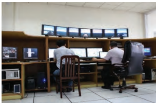
(b) Staff in control room
