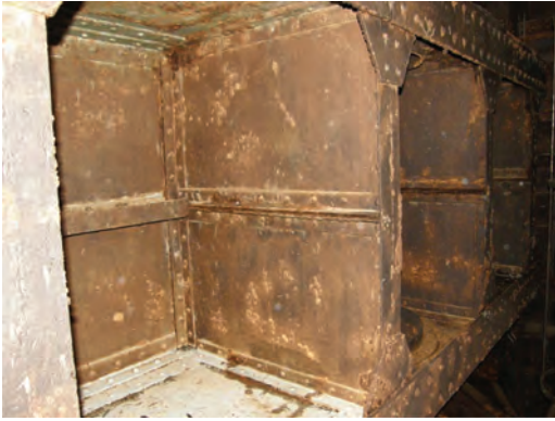
Figure 2. Deterioration of a steel cover plate.
