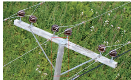
Figure 7. Wooden pole where a crack has been localized on the mast (see rectangle).
