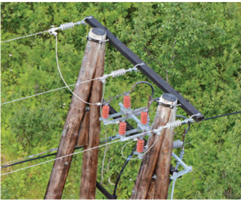
Figure 4. Third example of the shape of a wooden utility pole.
