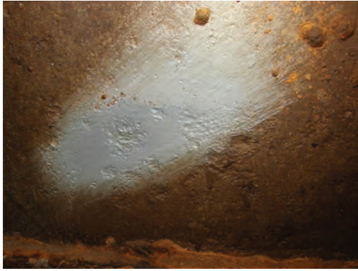
Figure 4. Pitting corrosion of a steel cover plate.
