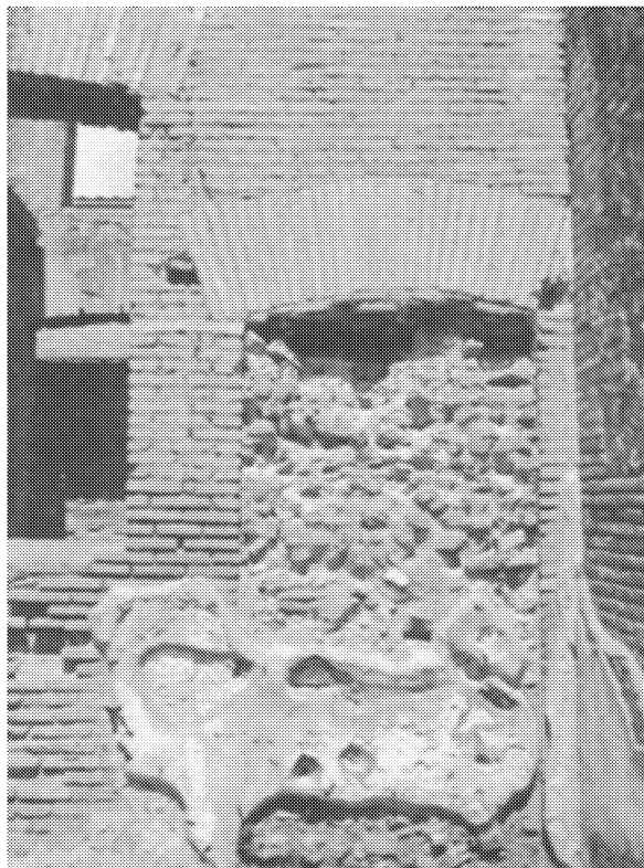
Figure 5.5 Rms 24/25, blocked doorway.
