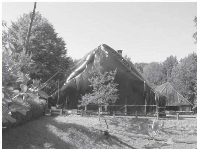
Fig. 4. Humidity-regulated warm-air method of house J1 in WFM Detmold.
