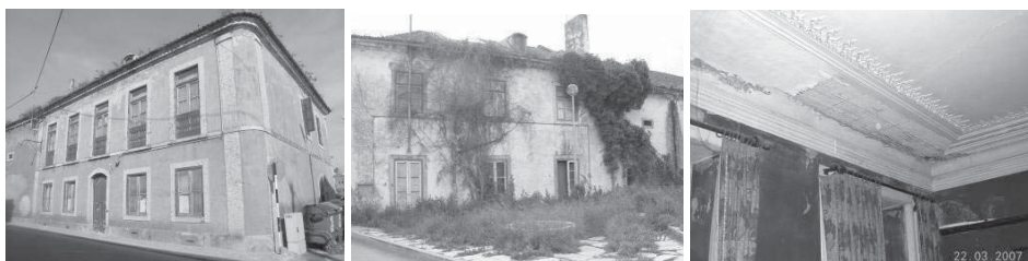
Fig. 1. (a) SW and SE facades of the building; (b) NE Facade; (c) Ceiling of a room in the 1 st floor.
