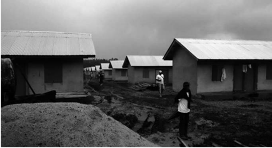
Figure 7.1: A new CDC camp under construction: laborer camps. Notice the well-aligned buildings.
