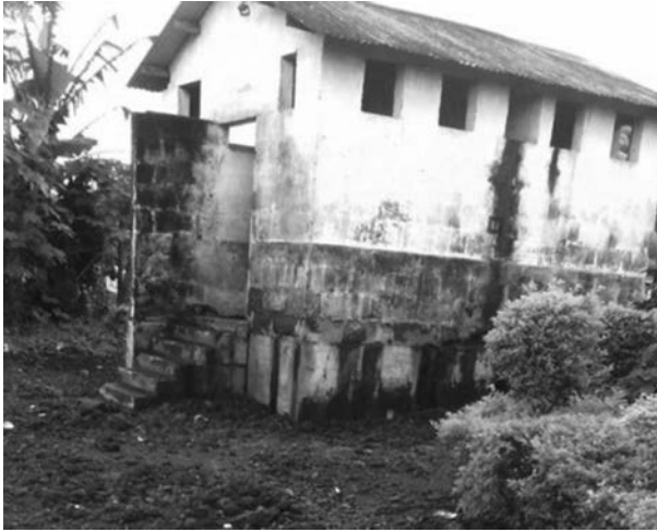
Figure 7.5: Communal bucket toilet, CDC Camp, Moliwe (notice the bucket-holding compartments at the base of the building).
