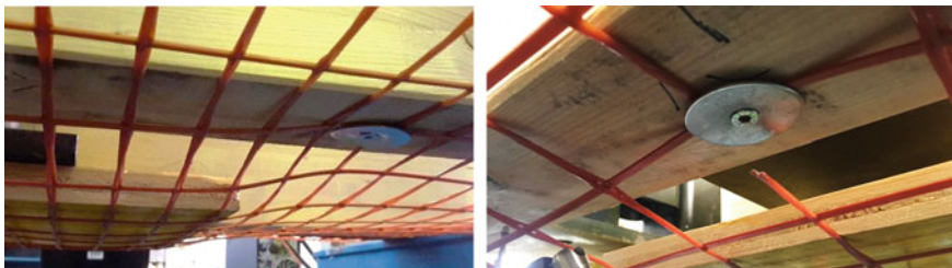
Fig. 8 Typical grid shear failure at anchor positions
