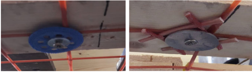
Fig. 3 Anchorage type: anchor with PE washer (left) and anchor with steel washer strengthened using a single mesh of 40 × 40 mm composite grid
