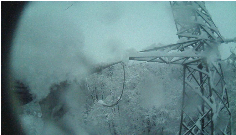
Fig. 6. Real state of a phase conductor - 18 January 2019
