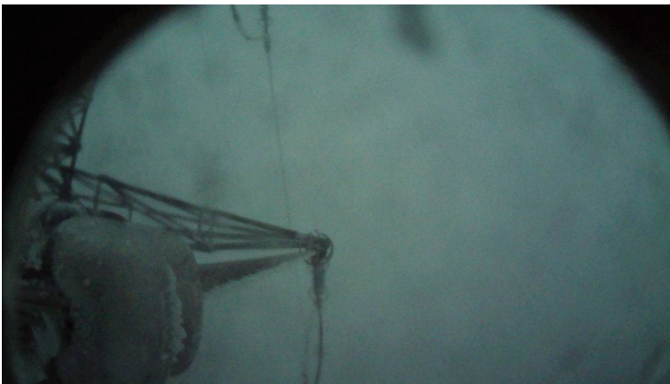
Fig. 4. Real state of a phase conductor - 20 November 2018
