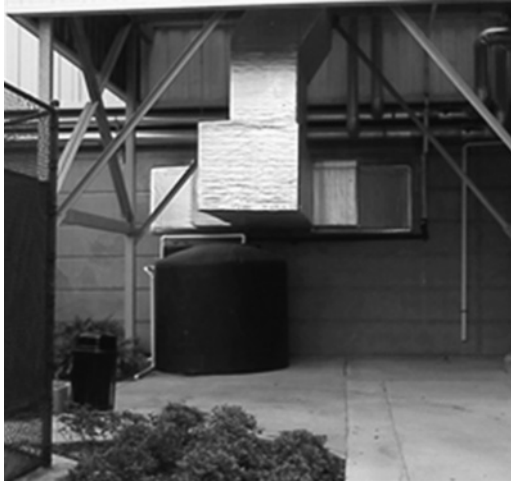
Figure 9.3 Condensate Storage at Bob Martinez Athletic Centre.
