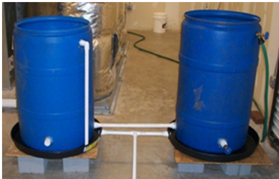
Figure 9.8 Condensate holding tanks and irrigation pump.
