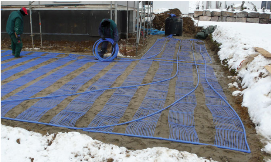
Fig. 3.8 A ground heat exchanger can be used for heating in winter and cooling in summer. Depending on its shape and depth, it is used for subsoil heat storage, and also for the extraction of geothermal energy. The thermal conductance depends on the ground water flow and many other site-specific conditions [28]
