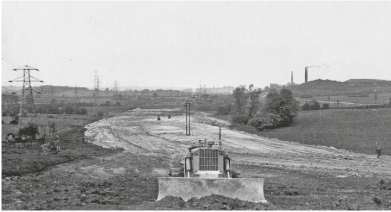
Figure 3.2 The construction of the M1 motorway through Bedfordshire in 1959 is marked by a swathe of bare earth, cleared and levelled by an army of machines such as the bulldozer prominent in the foreground. Source: photograph taken by Ben Brooksbank and reproduced by permission of the photographer.
