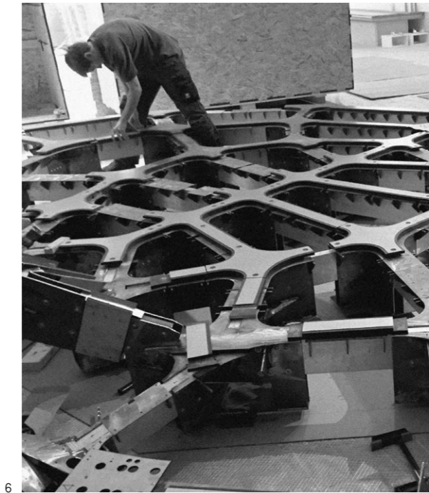
connection withstands live-loading and rotation due, in part, to compounding bolthole tolerances, resulting in a deflection effect in aggregate upon the canopy (Fig. 6).
