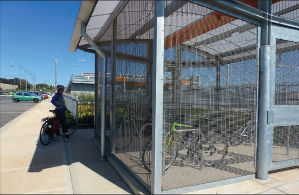
Figure 15.22: Access from the rear of the bicycle cage is unsafe. (Source: Author's own work.)
