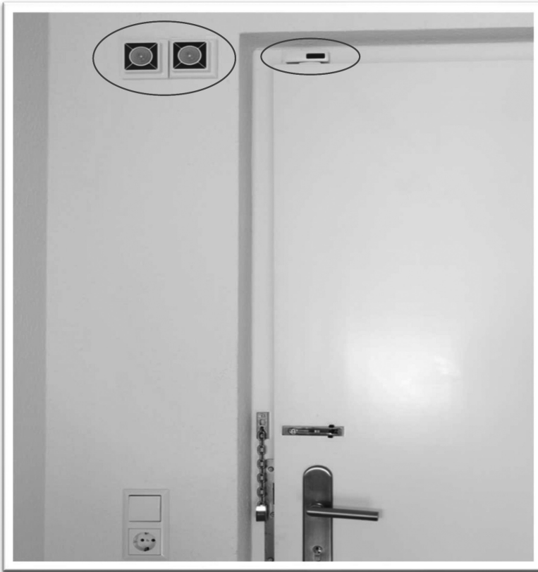
Figure 12.1 Door with motion sensor (left) and door sensor (right).
