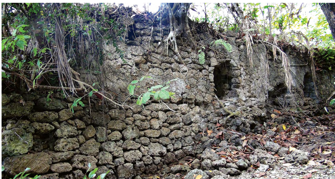
Figure 10.3. The thick, more than 2 m high lutur , or stone wall, that made up the base of mosque of the old Ujir village and which doubled as a fortification, located strategically at the water's edge.
