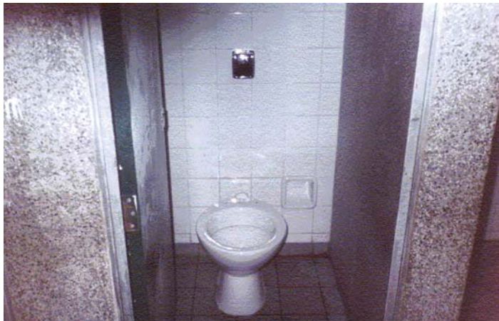
Figure 6.10 Replacement of automatic shut-off toilets. Source: Miya Corporation.
