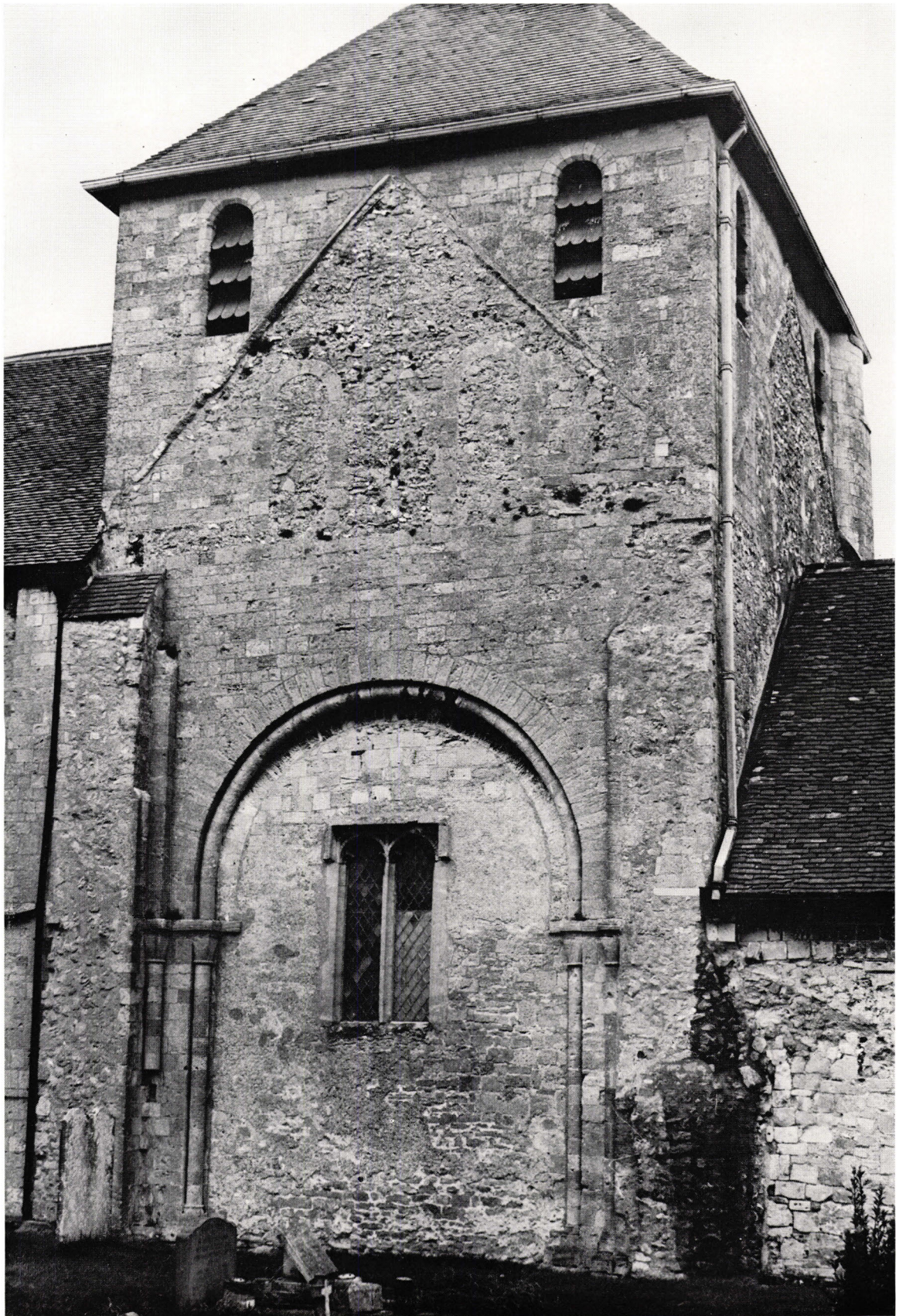
St. Mary's Church: face of south wall showing the abutment of the demolished south transept (photo: David Baker)
