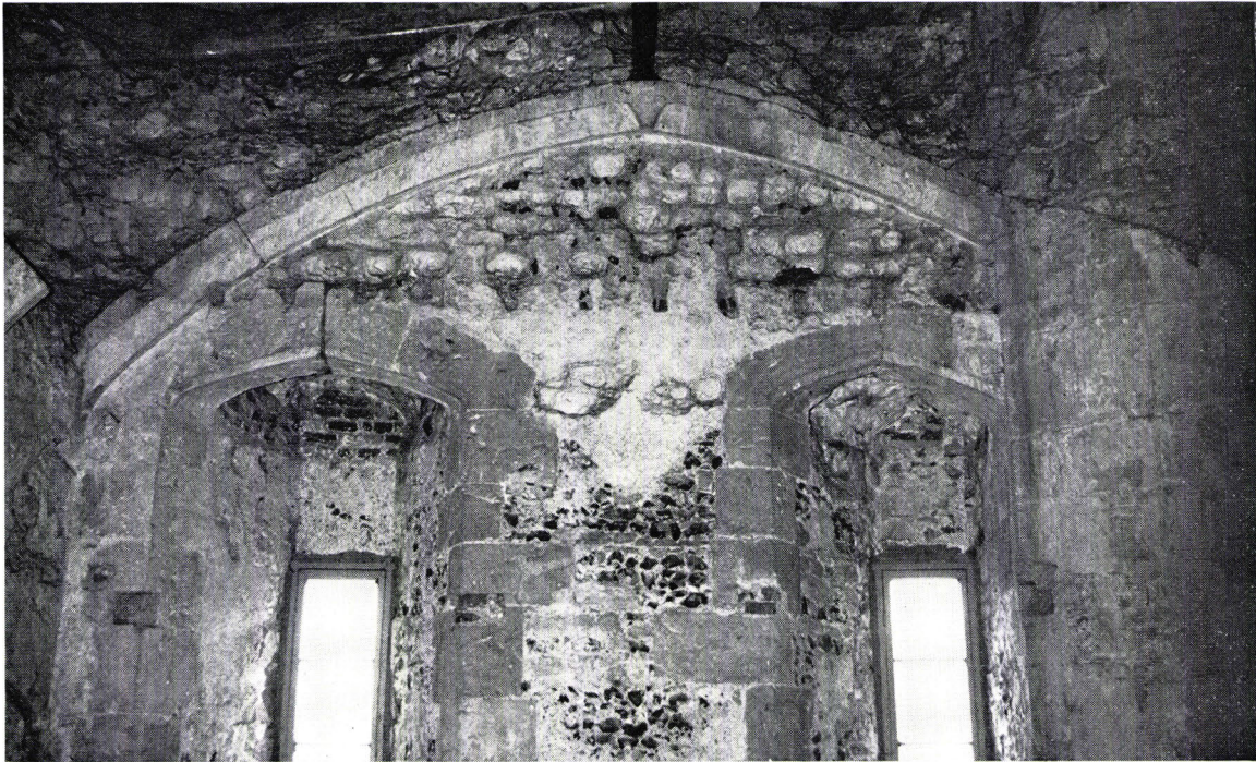
a. The landgate: upper chamber showing inside of west wall (photo: Mike Rouillard)
