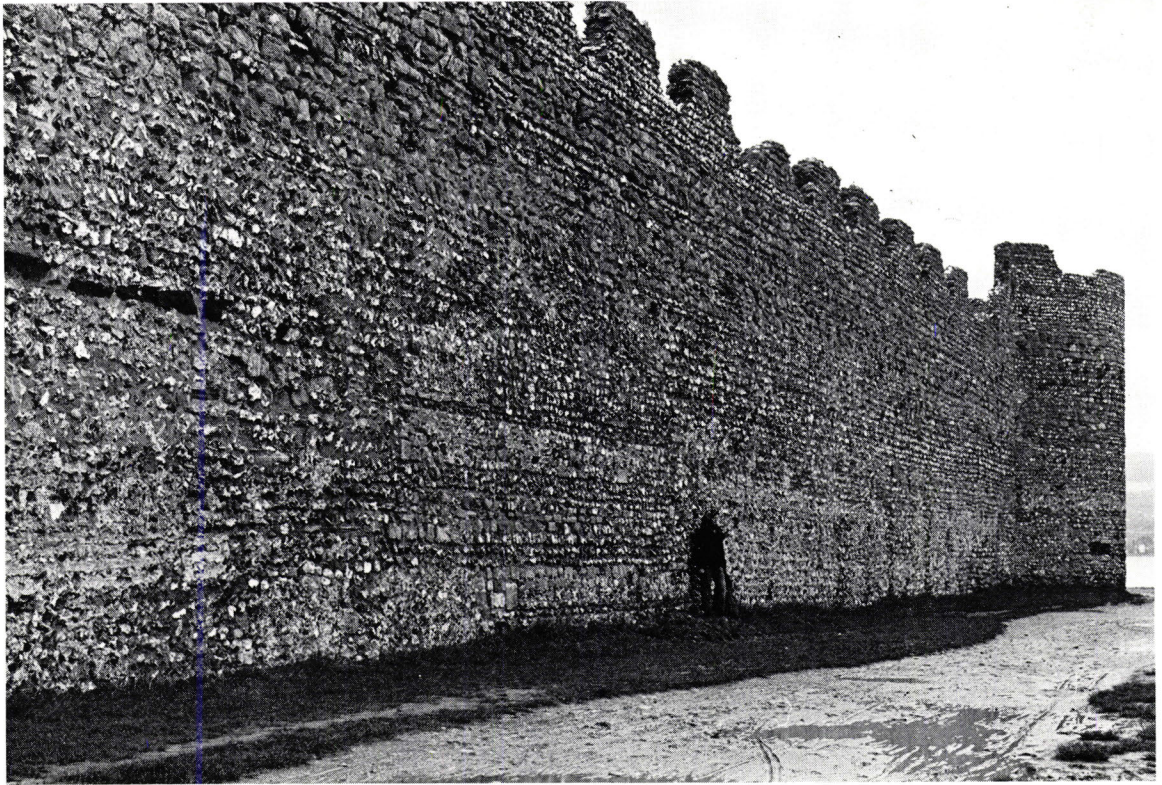
a. The east wall of the Roman fort: the outside refaced in medieval times (photo: David Baker)
