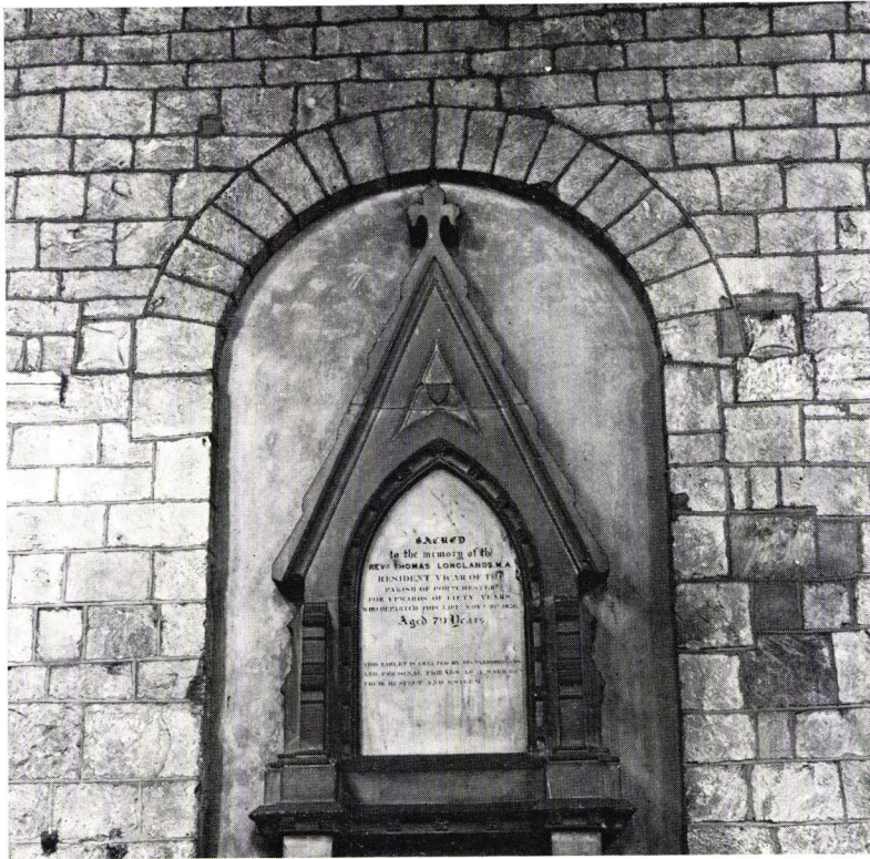
a. St. Mary's Church: blocked doorway in the north wall of the nave (photo: Mike Rouillard)
