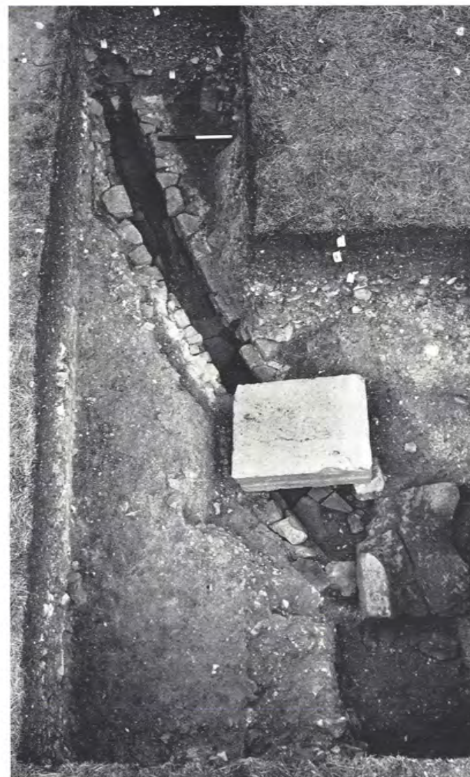
(c) the drain passing from the courtyard beneath one of the stylobate blocks still in position; looking east (p. 117)
