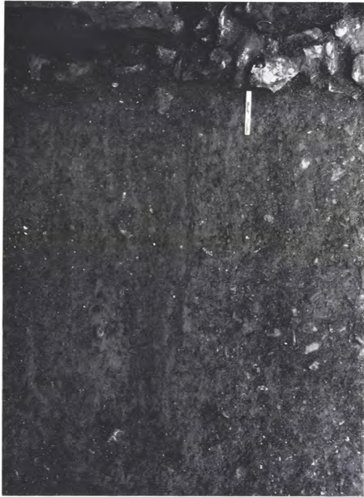
a. Rotted sill beams for north wall of Timber Building 4; vertical view (p. 47)
