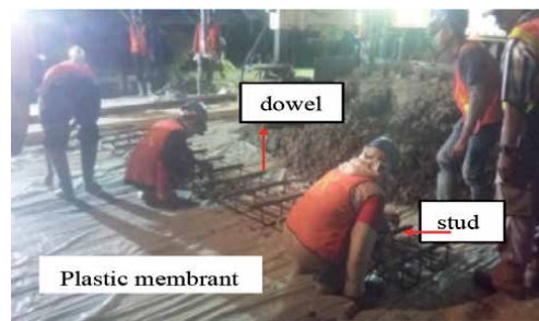
Figure 8. Dowel baskets placed on an LC. Red line: Dowel. LC: Lean concrete.
