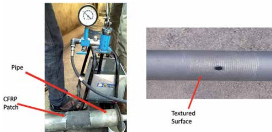
Figure 9. Pipe hydrostatic pressure testing (left side) and surface prepared before patching (right side).
