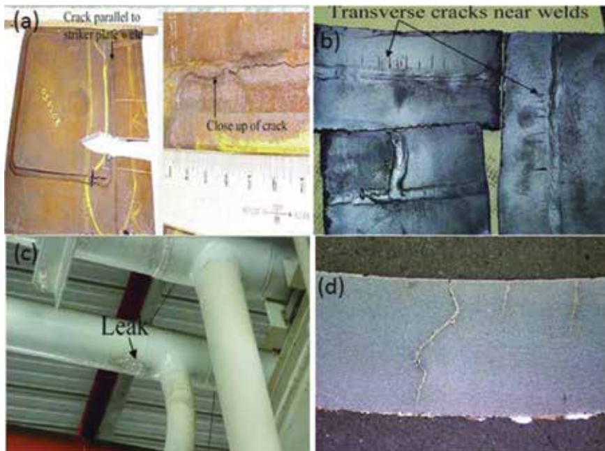
Figure 4. SCC failures showing (a) SCC in steel tank bottom, (b) SCC in steel air eliminator vessel, (c) leak in piping resulting from a crack adjacent to the weld, (d) multiple crack initiations and through-thickness propagation in piping [8, 16].
