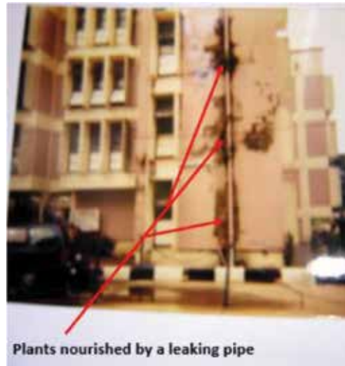
Figure 1. Part of a 2-year-old engineering faculty building at one sub-Saharan Africa's university (author).
