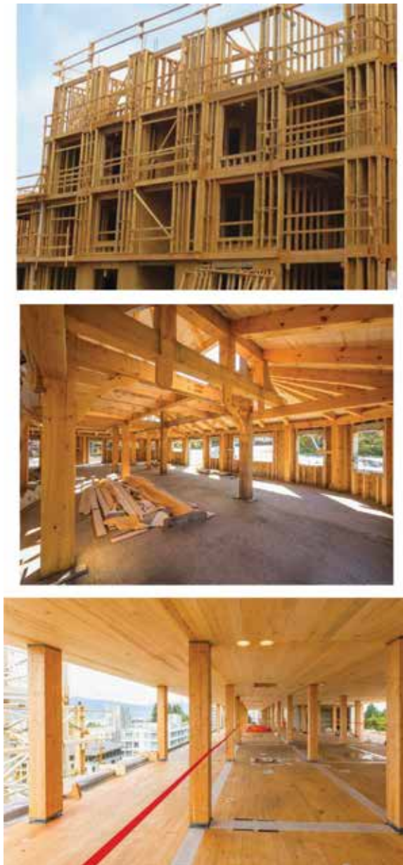
Figure 2. Wood building construction methods. Top: Light-frame construction (Source: Photo obtained from Okoye et al. [5]). Center: Post-and-beam construction (Source: Photo obtained from Post & Beam Homes). Bottom: Mass timber construction (Source: Photo obtained from UBC Public Affairs).
