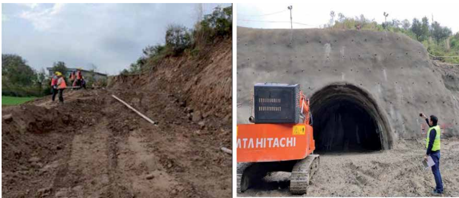
Figure 4. A view of the construction of approach road in the left for the tunnel shown on the right.
