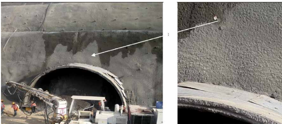
Figure 10. Bireflex targets fixed at a tunnel portal to monitor the movement of the slope.
