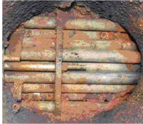
Figure 4. Oxides of corrosion in the tubes of a heat exchanger (H&C Heat Transfer Solutions Inc. 2013).
