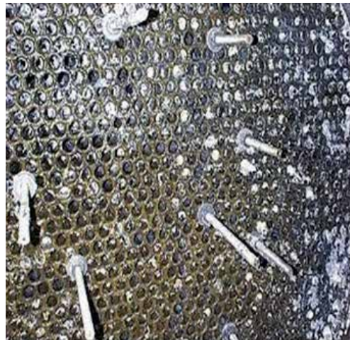
Figure 5. Icy icing of polymer products in a heat exchanger (Source: By courtesy of H&C Heat Transfer Solutions In.).
