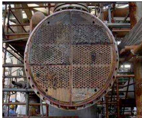
Figure 2. Tubular heat exchanger in maintenance due to the presence of biofouling in its tubular bundle (Source: By courtesy of Merus-the water conditioner company).
