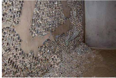
Figure 1. Presence of mussels in the water box of a condenser (Source: By courtesy of Nuclenor).
