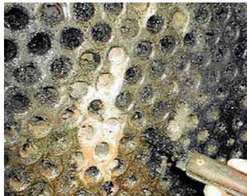
Figure 3. Residue of hydrocarbon in the tubes of a heat exchanger (Source: By courtesy of H&C Heat Transfer Solutions Inc. 2013).
