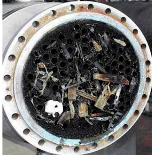
Figure 7. Accumulation of solid particles in the plate of a tubular heat exchanger (Source: By courtesy of AH&C Heat Transfer Solutions Inc.).
