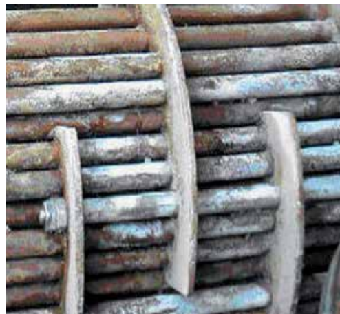
Figure 6. Precipitated salts in the tubes of a heat exchanger (Source: By courtesy of H&C Heat Transfer Solutions Inc).
