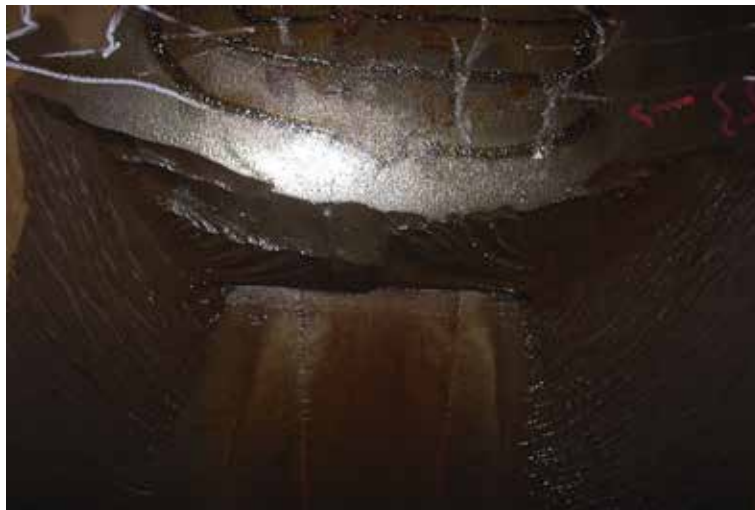
Figure 7. Typical spalling of component result from contact fatigue.
