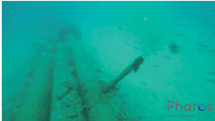
Figure 20. Detail of the diffuser system of the submarine emissary pipeline.
