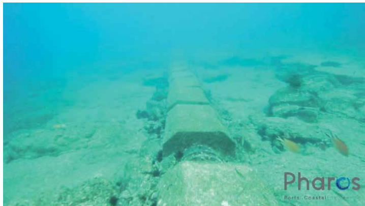
Figure 22. Detail of the concrete weights in a pipeline section near the coast.
