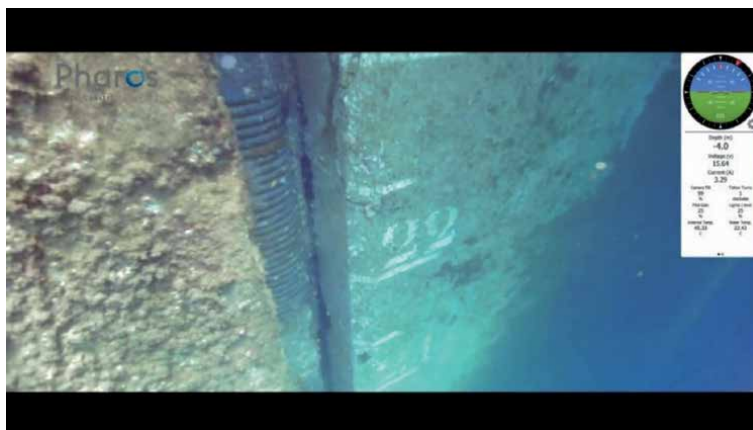
Figure 17. Detail of depth markers on the facing of concrete quay blocks and joint.
