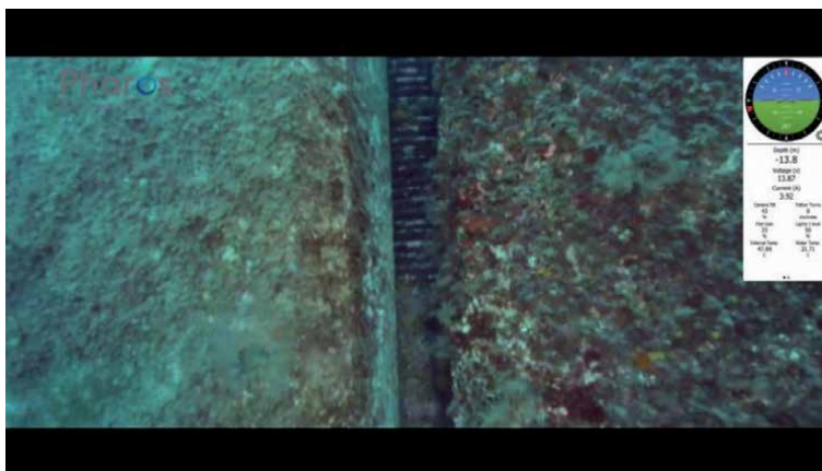
Figure 12. Detail of joint between concrete quay blocks in vertical face.
