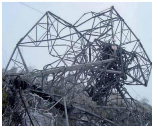
Figure 3. Transmission tower collapse caused by ice accumulation.
