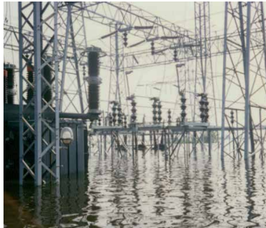
Figure 1. Flooded substations during the 1993 flood at UE.
