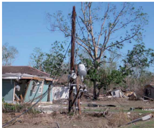
Figure 2. Damage to the electric distribution grid near Pt. A La Hache, LA.
