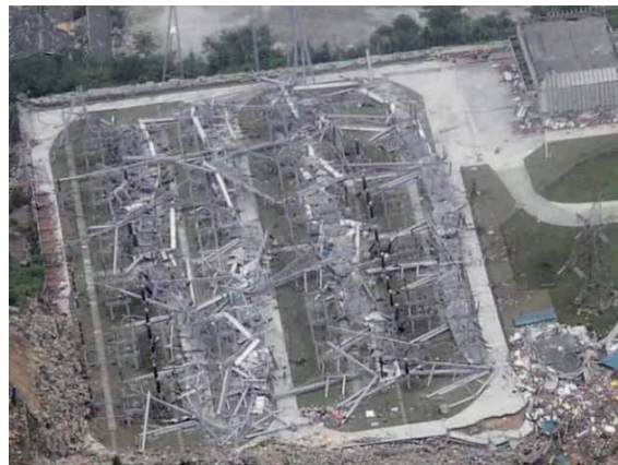
Figure 4. Damage to equipment in the Ertaiشان switchyard.
